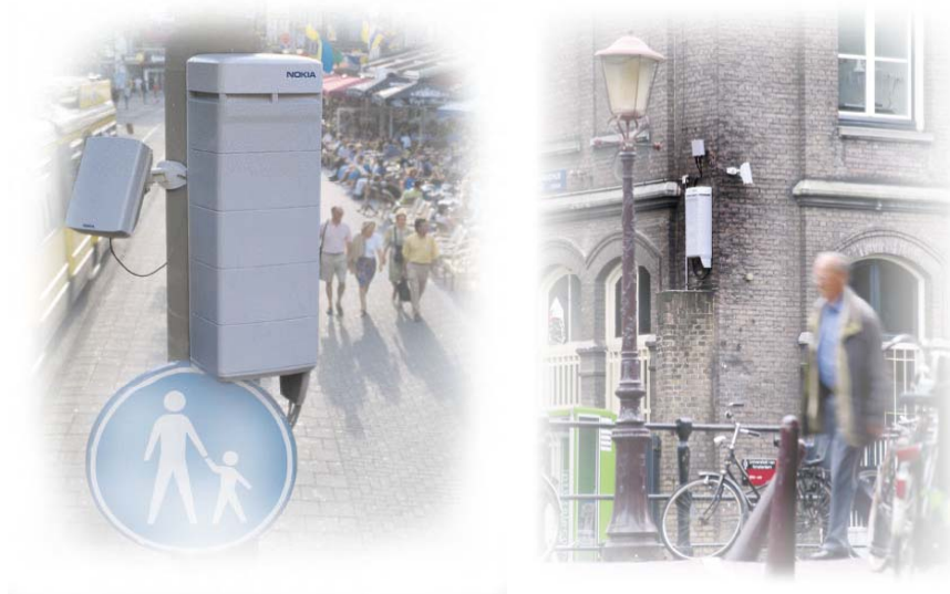
Figure 6. Nokia MetroSite Base Transceiver Station
